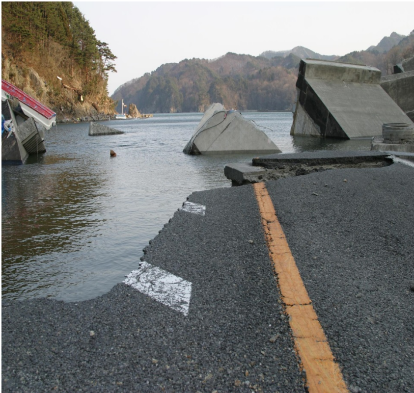
OTSUCHI ROAD DAMAGE, Iwate Prefecture
